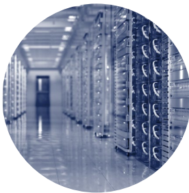
Data centre thermal management
